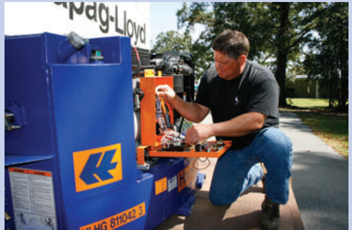
A service technician conducts diagnostics on one of Hapag-Lloyd’s generator sets during an annual SeaCare Solutions preventive maintenance check-up.
