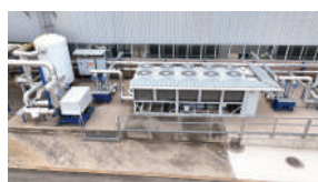
30KAV air-to-water chillers
