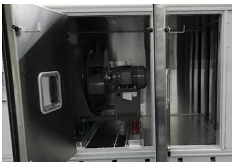
Corrosion Resistance Material
