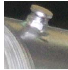
Purge and Vent Valves
